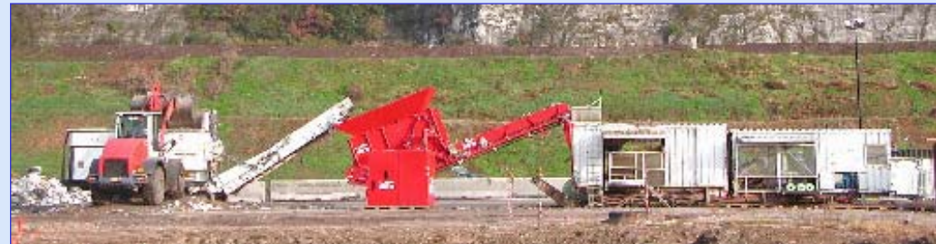
Example baling process EuRec®-Shredder > EuRec®-Bunker > EuRec®-RBS System
